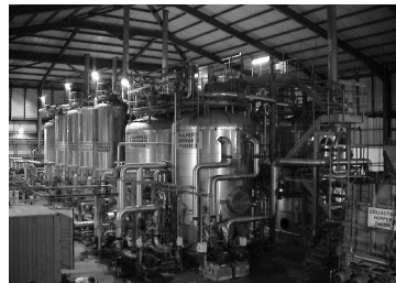
Cambi 8-reactor THP plant for treatment of sewage sludge from Ringsend Sewage Treatment Works, Dublin, Ireland, with a capacity of 1.2 million p.e., 36,000 tonnes dry solids; 3 x 4,500 m 3 digesters; 45,000 m 3 per day of biogas; 4 MW electricity production; final product: granulated and dried fertilizer
